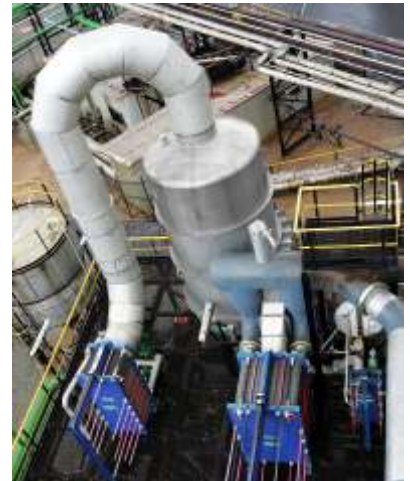
The Alfa Laval Services equipment installed at the AEL
